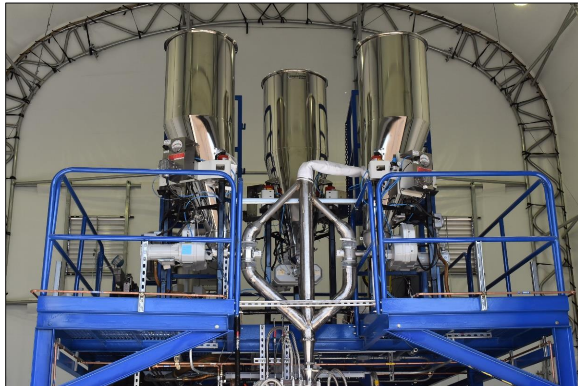
2" stainless steel pipe for pressure relief 1 um filter sock to reduce dusting
